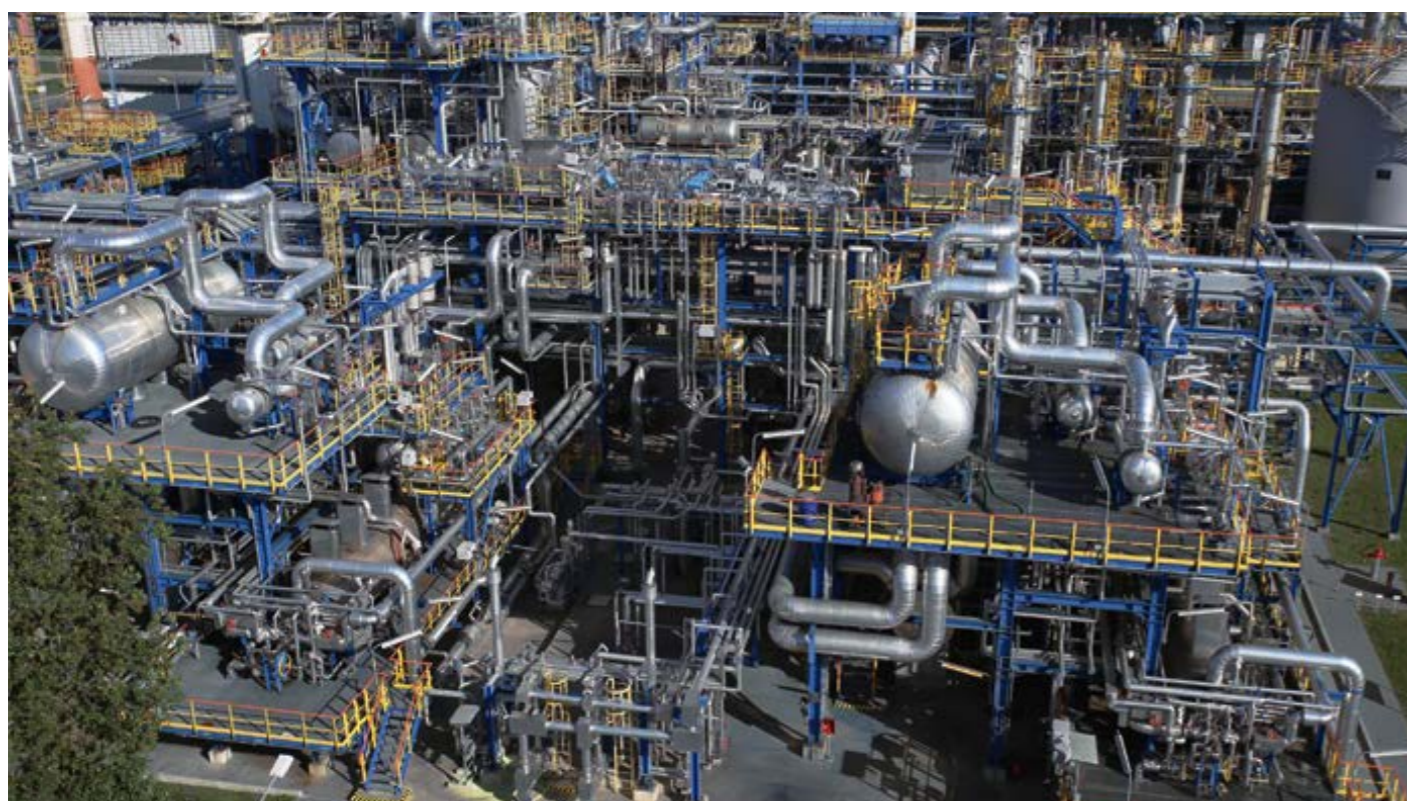
Two of the four Claus units at the Polish refinery in Gdansk that are being engineered for increased capacity through oxygen enrichment.
