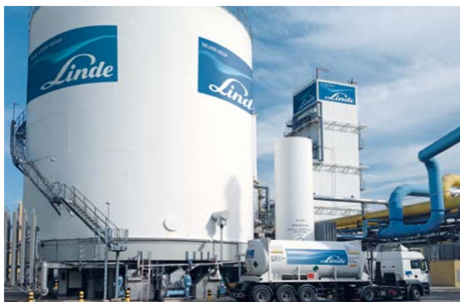
Liquid Air Energy Storage (LAES) tank at an air separation plant in Leuna, Germany.
