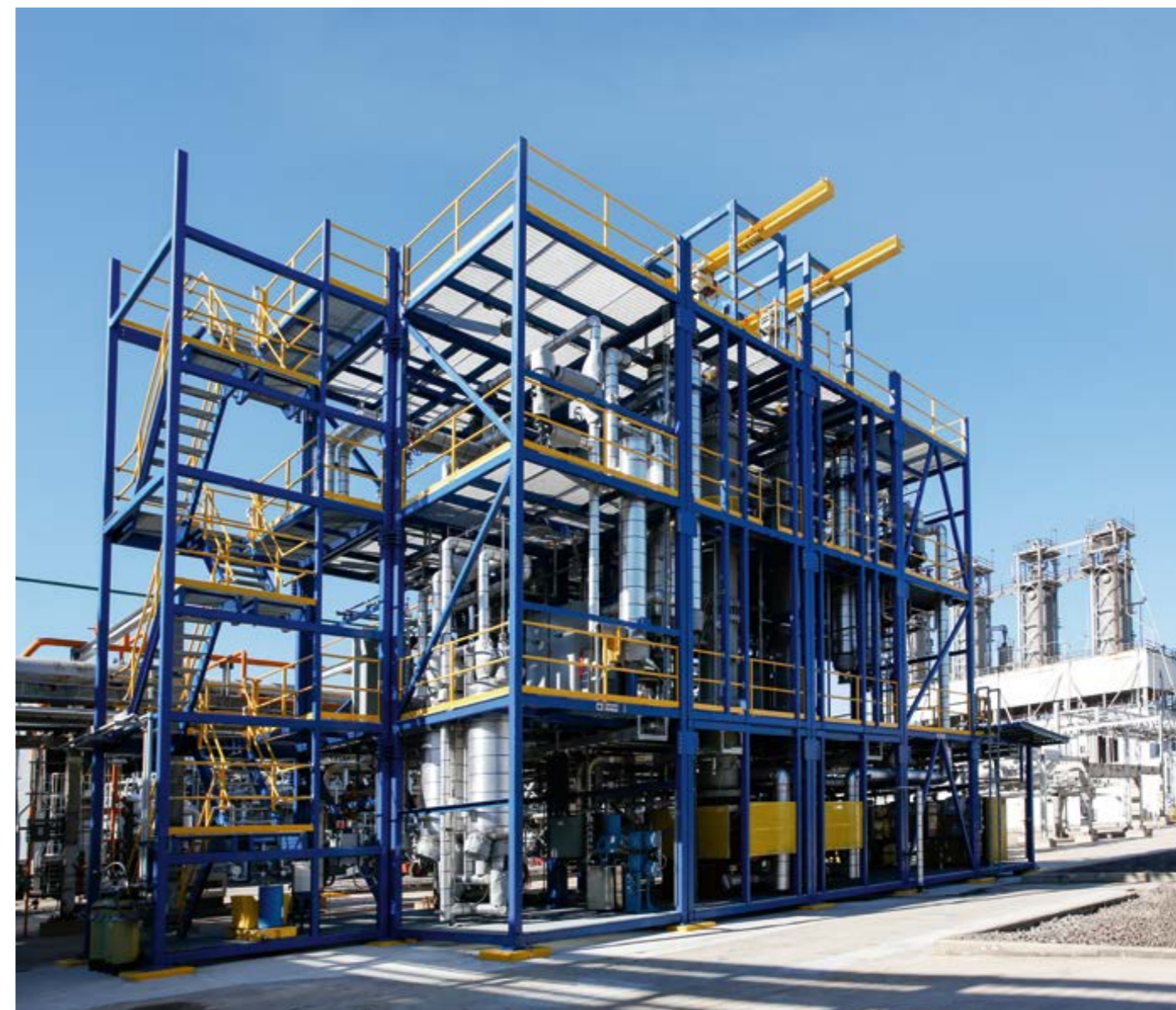
Highest value creation: Oxidative Coupling of Methane (OCM) pilot plant in La Porte, USA.
