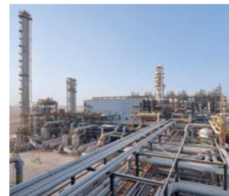
Ethylene production facility delivers a total capacity of 4.5 million tonnes per annum.
