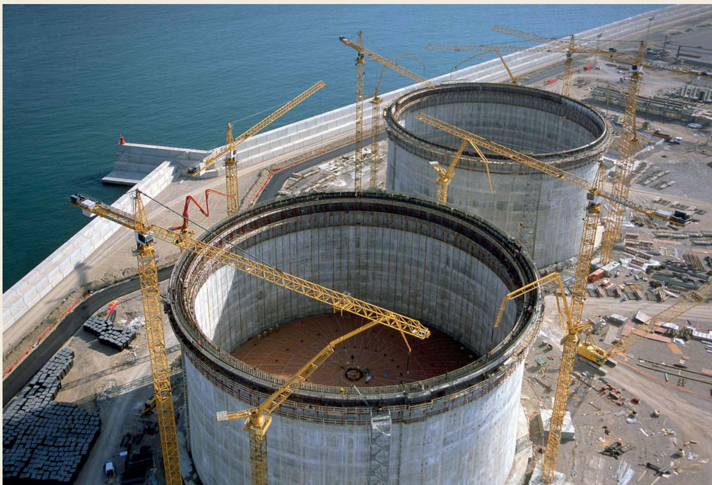
Construction of pre-stressed concrete outer tanks (image courtesy of STRABAG International GmbH)
