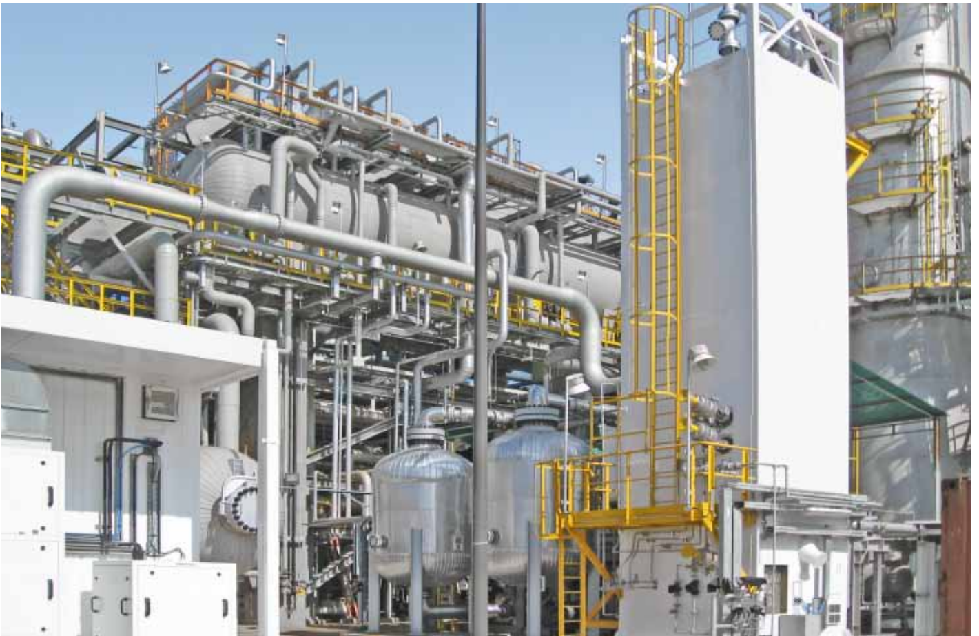
Hydrogen recovery from the purge gas stream generated by an ammonia synthesis plant in Moron, Venezuela.
