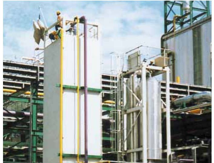
Hydrogen recovery from the purge gas stream generated by an ammonia synthesis plant in Palembang, Indonesia.
