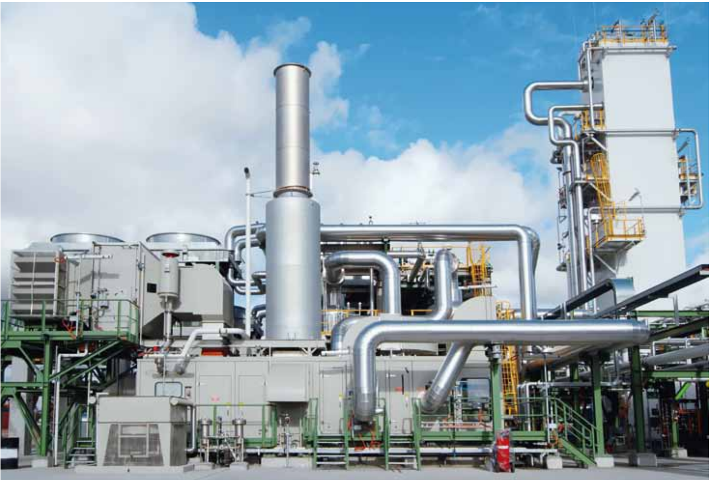
Gas turbine driver for MRC compressor.
