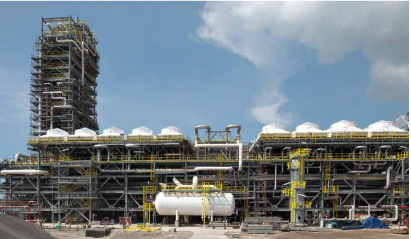
Mid-scale StarLNG® plant with up to 0.8 mtpa liquefaction capacity in Bintulu, Malaysia.
