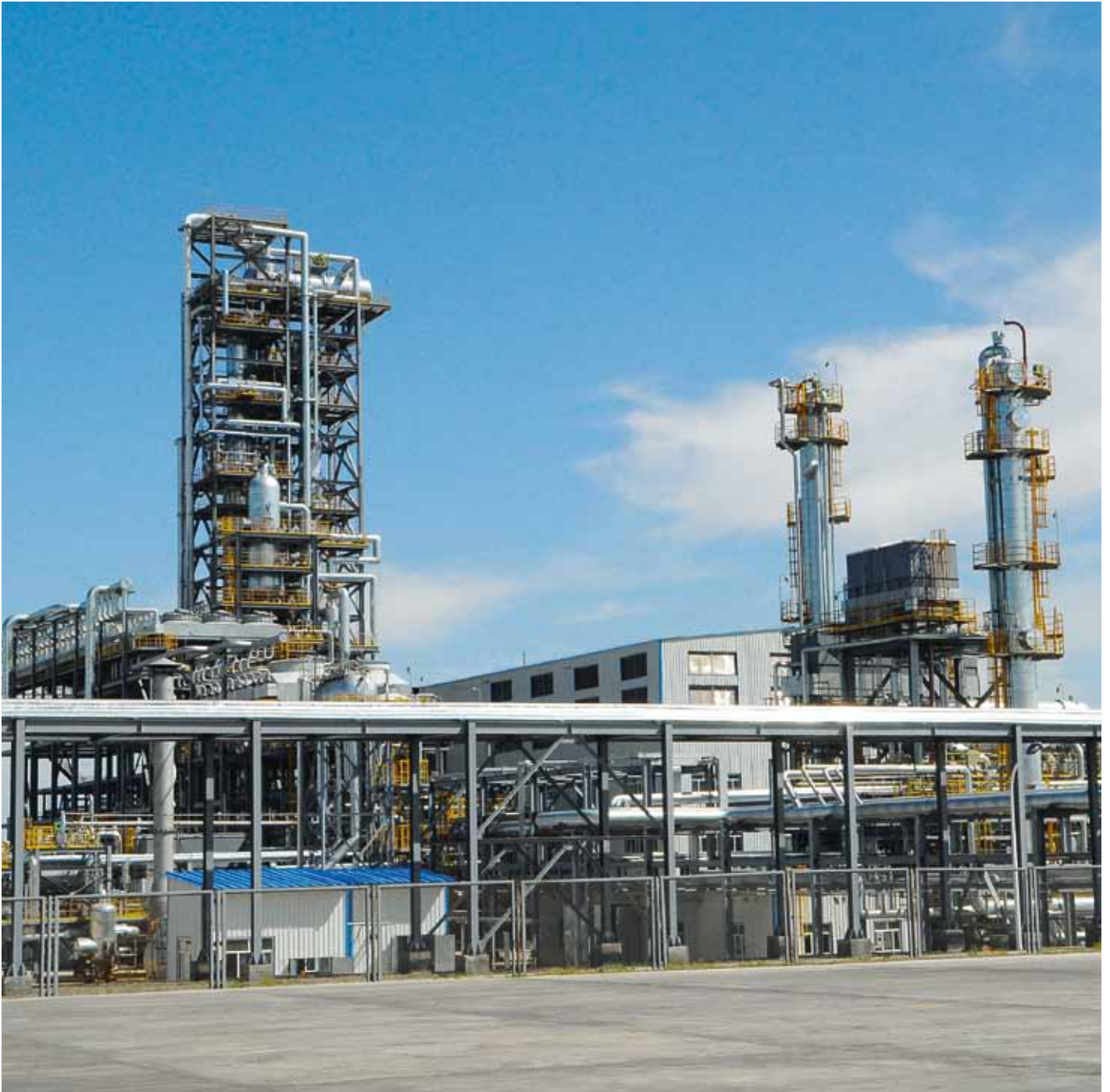
Mid-scale StarLNG plant with 1,200 tpd liquefaction capacity in Jimunai, China.
