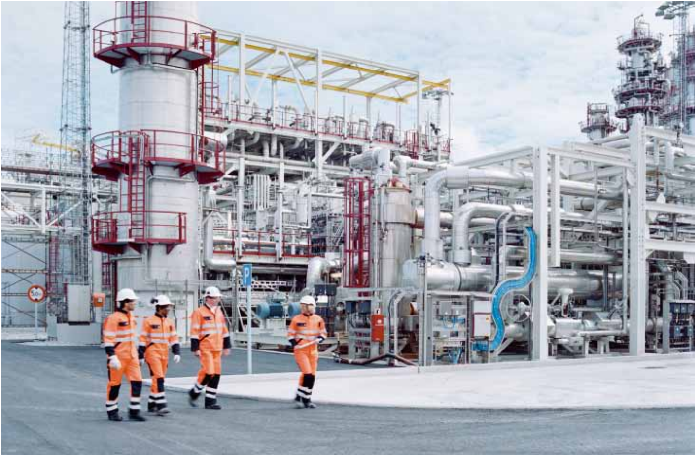
LNG plant at Hammerfest, Norway.
