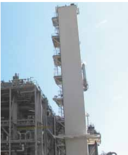
Nitrogen rejection unit (NRU) in Karratha, Australia.
