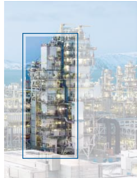
NRU integrated in LNG plant at Hammerfest, Norway.
