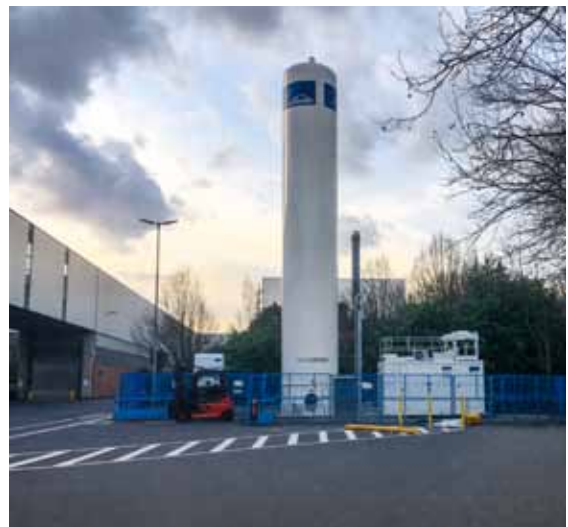
Fuel cell forklifts fueling station
